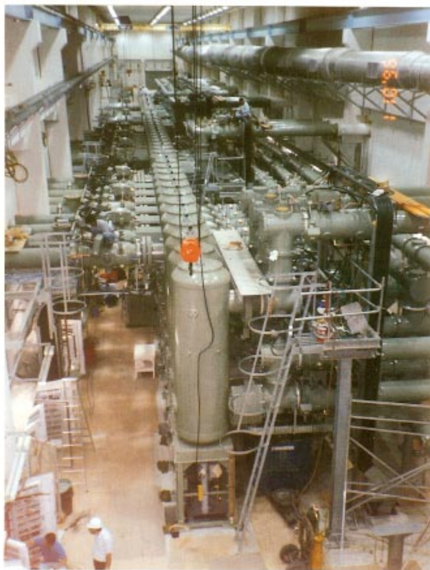
380 kV Gas insulated switchgear building
